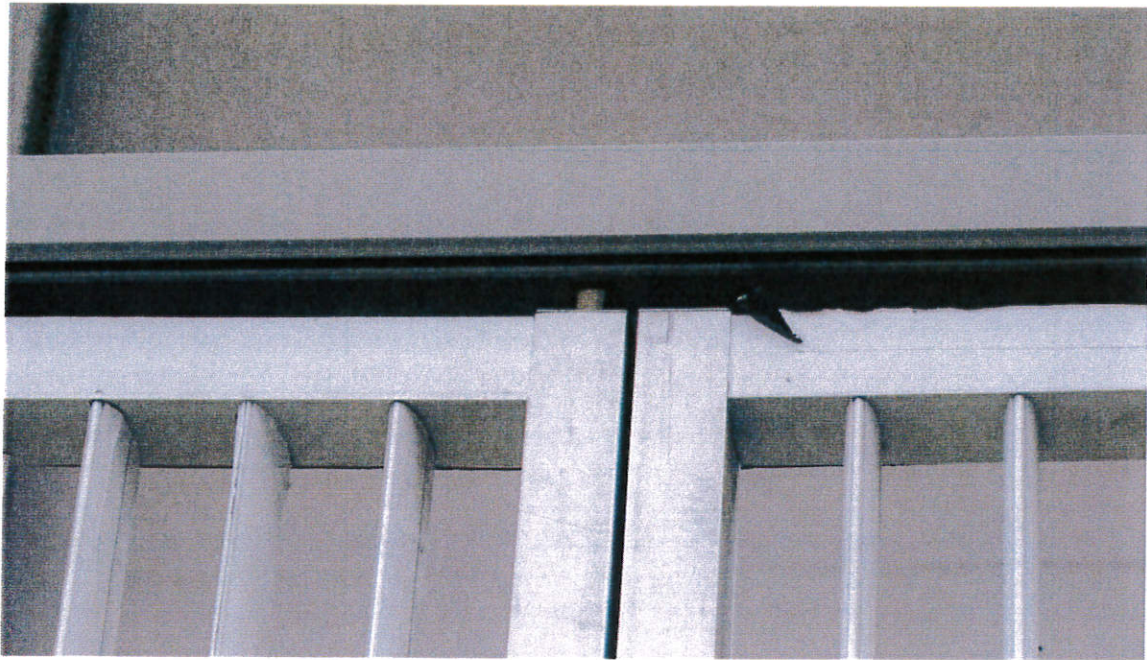
Figure 4: Damage observed on Lock Bar
